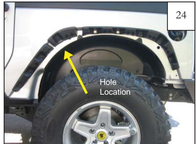
Secure inner piece D8 (and P8 for passenger side installation) to the sheet metal using the following 2 STEPS: Step 1 Position inner piece on fender, aligning with existing factory hole in sheet metal.
